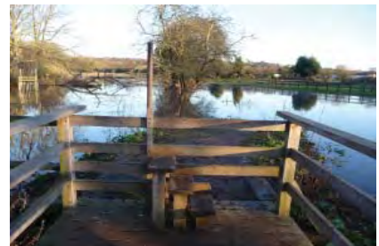
The footpath between the Hammerton's and Douglas Meadows boardwalk regularly floods on high tides
