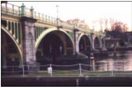
The fine arches and technical innovation of Richmond Weir, restored for its 1994 centenary by the PLA
