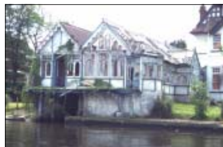
Domestic boathouses add a special character to the waterfront - albeit a vulnerable one
